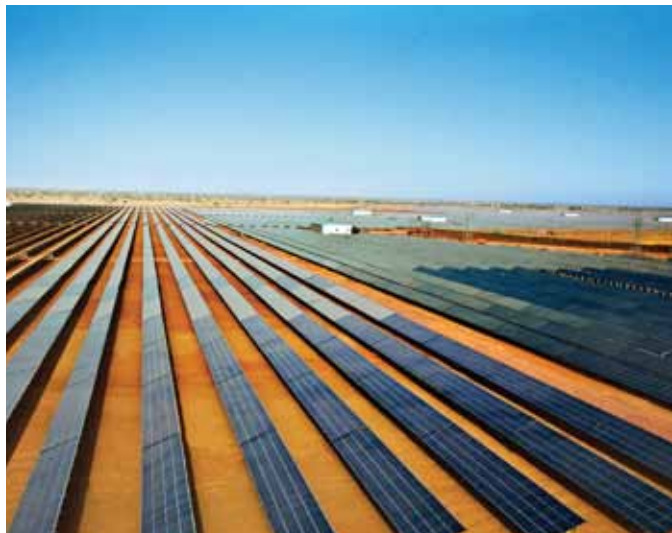
Dhursar I Rajasthan 40 MW Solar PV
